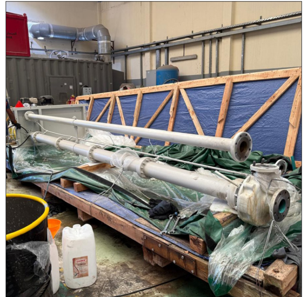
Internal surfaces following ZERUST® Axxaclean® 2048 Cleaning Solution and ZerioGuard® 5 treatment
